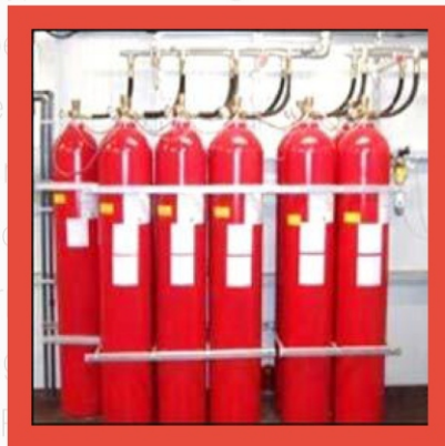
CO2 Flooding System
